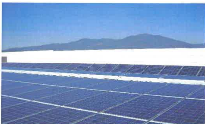
Nau CT Solutions, Barcelona – 24,84 kWp
